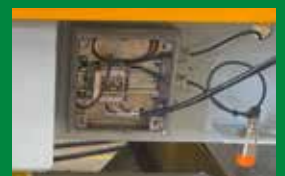
Proximity sensing for gate position
