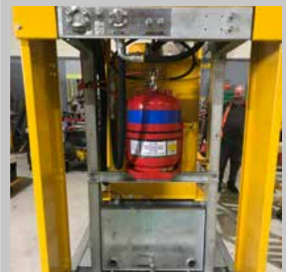
Fire Suppression System
