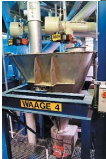
Mixing system for batch operation
