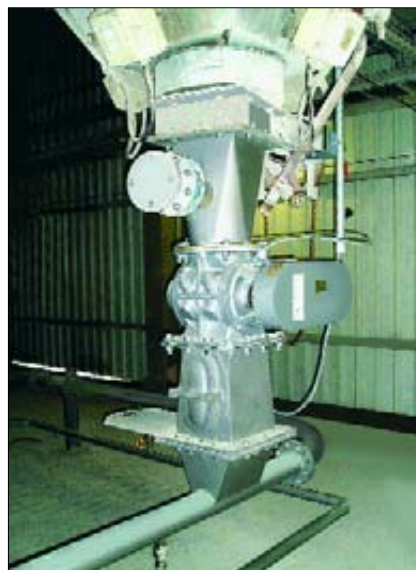
FLUIDCON transport system at E-on Farge Plant
